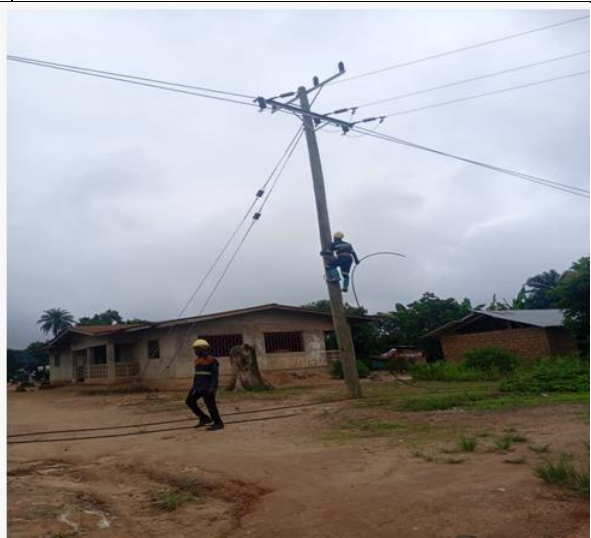
Bare overhead wires observed over private residential houses in Honeyahun, Kolahun District
