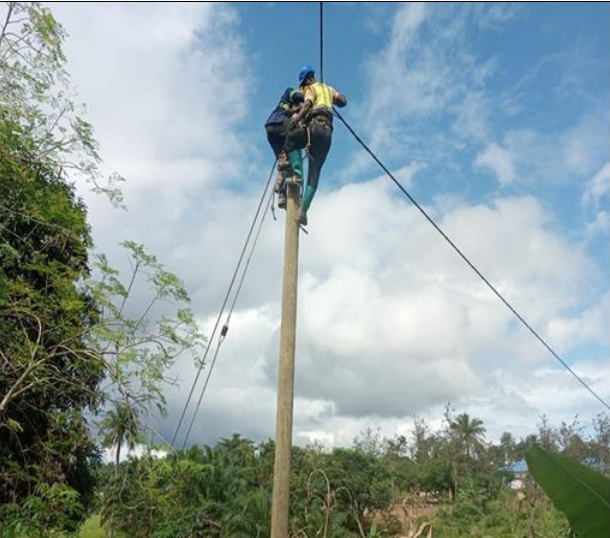
Replacement of bare wires with insulated cable in Johnny Town, Voinjama District.
